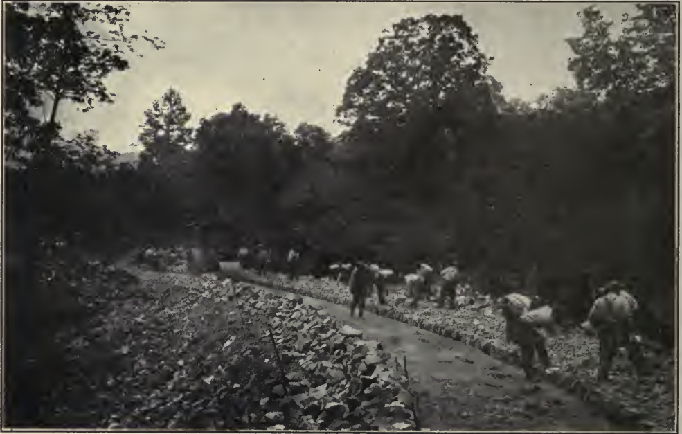
LAYING THE TELFERD BASE OF A BITUMINOUS MACADAM PAVEMENT IN A HEAVILY TRAVELED SECTION OF THE INTERSTATE PALISADES PARK RESERVATION, NEW JERSEY
